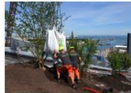
The root balls of the shrubs are supported by specially shaped reinforcement steel meshes.
